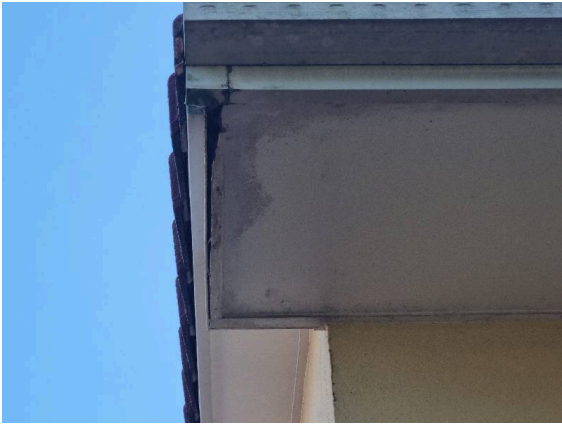
Example of fungal decay and water damage to eaves at unit 2.
