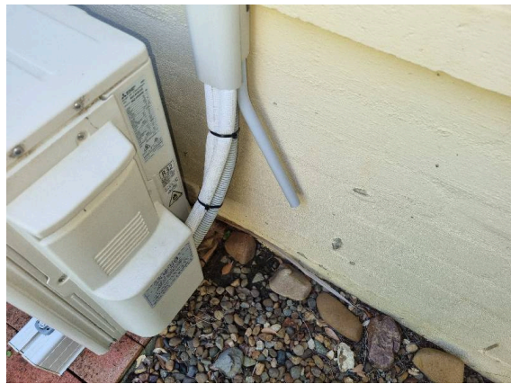
Example of air conditioning condensation pipe not connected to drainage which may allow for moisture buildup next to property which may attract termites.
