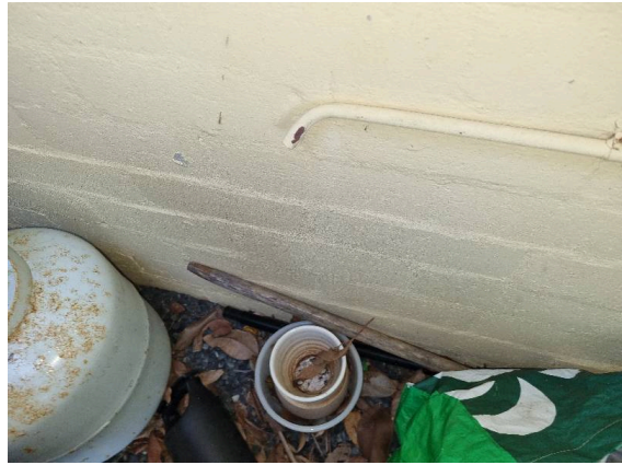
Example of hot water system overflow not connected to drain which can allow moisture to buildup next to property which may attract termites.
