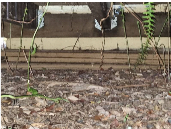
Example of stored timber in direct ground contact under rear deck of unit 4, which may attract termites.
